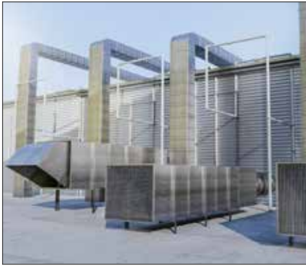
Air Handling Units
